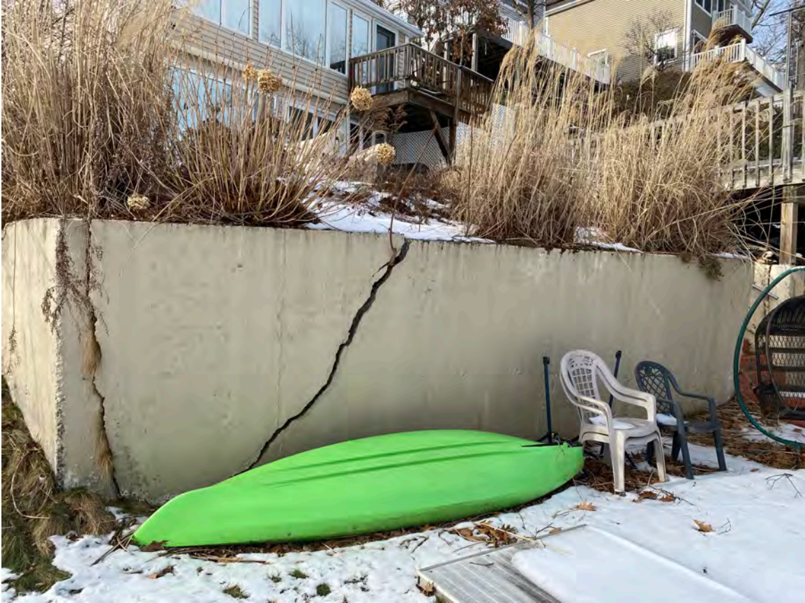
Picture Above: Large crack on front of wall and separation from south side existing concrete wall
