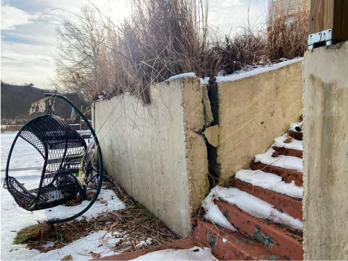
Picture Above: Large crack, existing wall leaning forward
