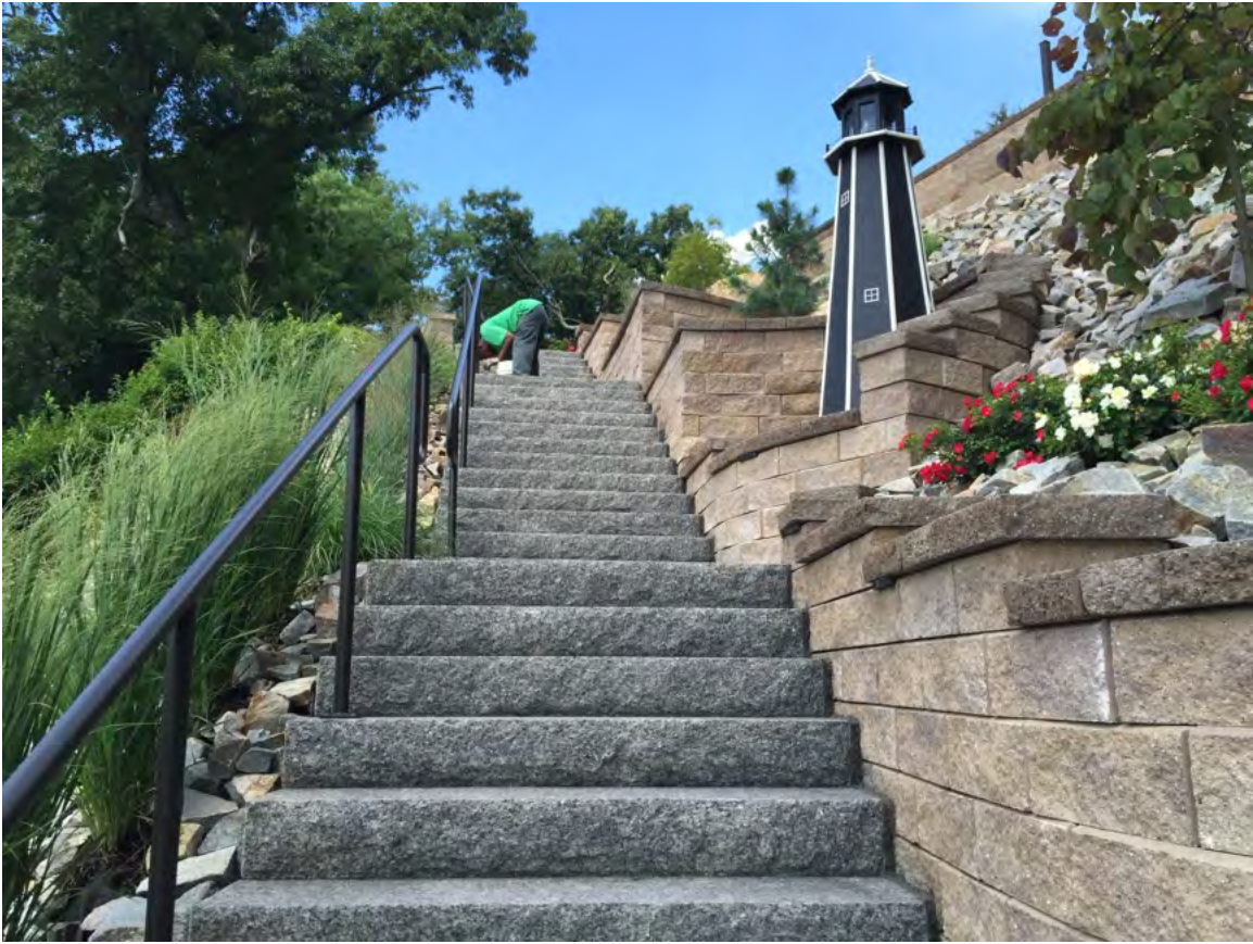
Picture Above: Installed Granite Steps by The Green Machine on Middle Pond
