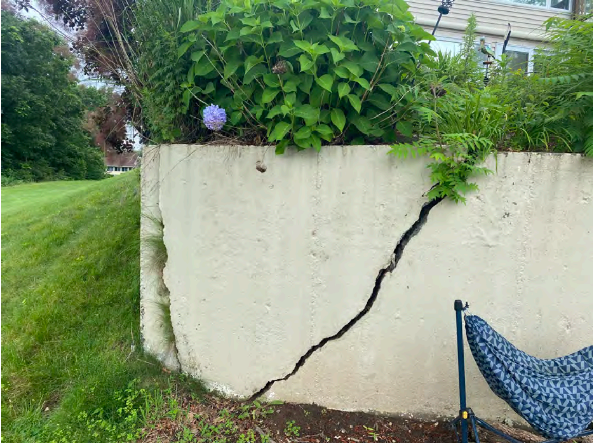
Picture Above: Close up of large front crack
