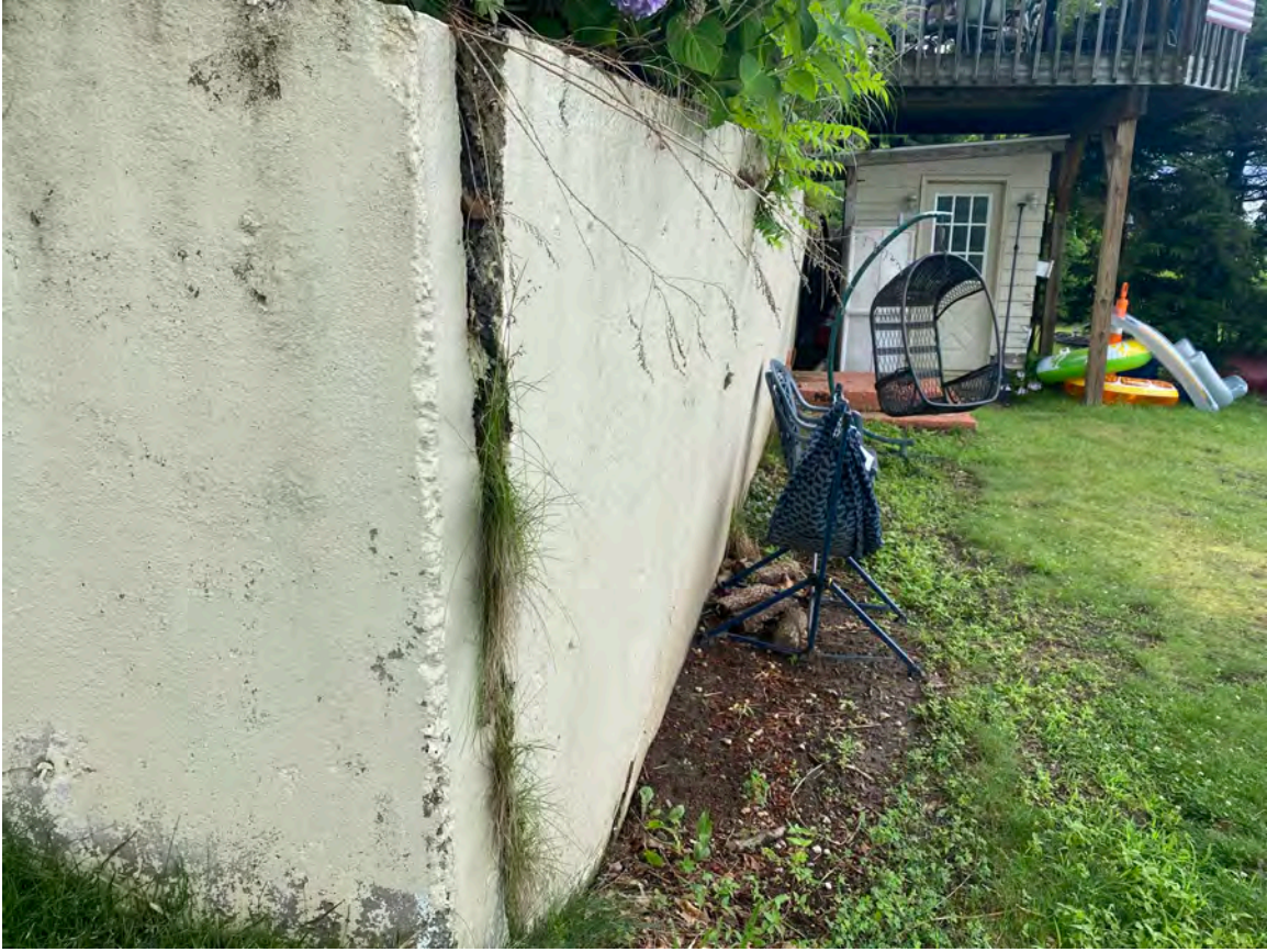
Picture Above: Close up of separation from south side existing concrete wall, existing wall leaning forward
